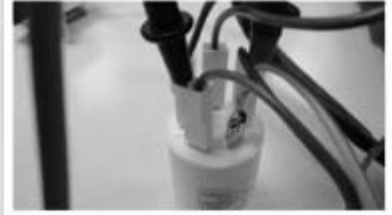
Picture F13-1: 220VAC control on L-N ends of the noise filter
