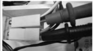
Picture F13-4: 220VAC control on outlet ends while On-off key is pressed
